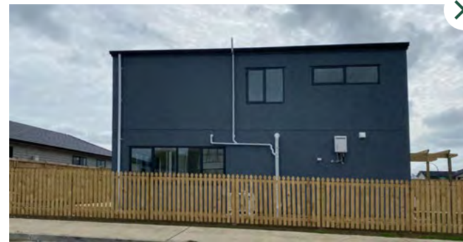
Pipes and accessories are all in a contrasting colour to the side wall of the house, and highly visible from the street.
